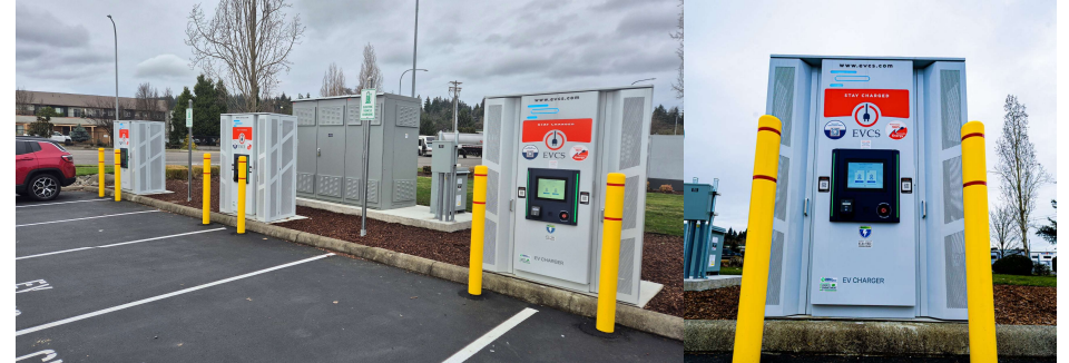
Cable Arm Protection, Market, WA USA
