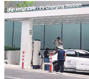
Hyundai E-Pit Station (Thailand)
