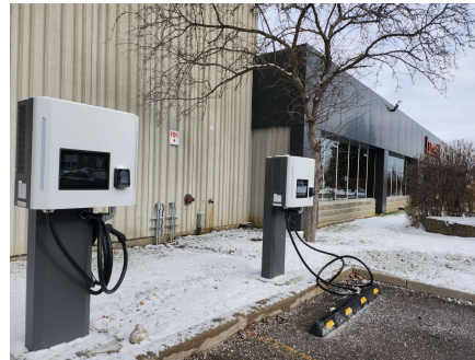
Enersaving, Richmond Hill CANADA
